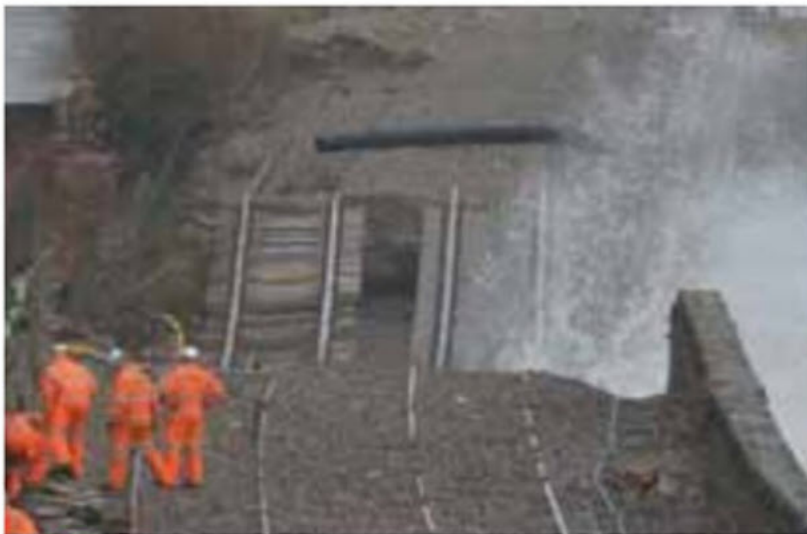
◀ Figure 23 The coastal rail line at Dawlish was destroyed by the winter storms of 2014.
