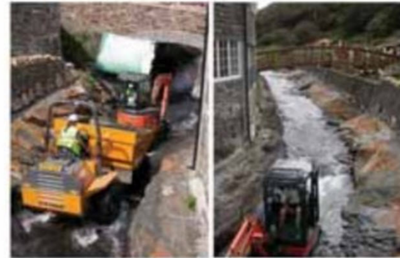
▲ Figure 19 Workmen using a JCB to dig out the rocky bed of the river under the main bridge during 2007.
