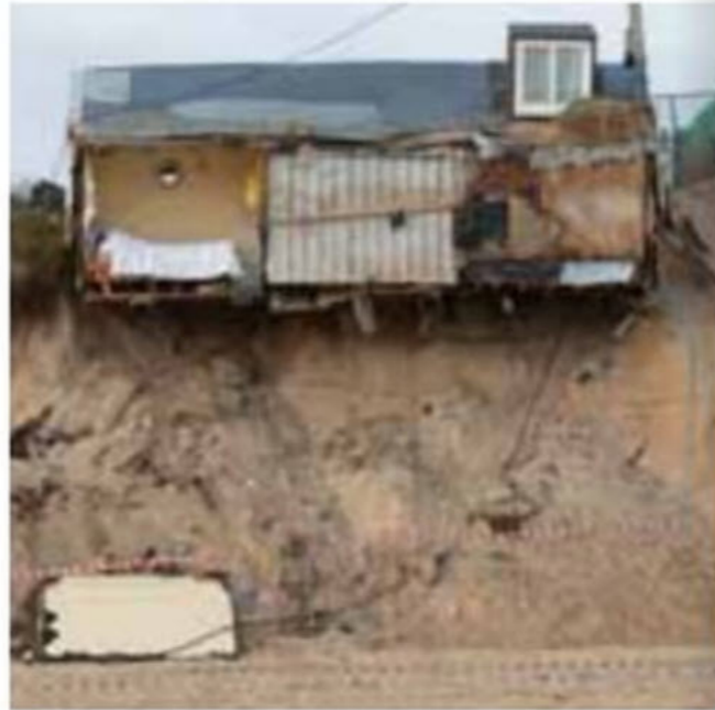
▲ Figure 5 Rapid coastal erosion of the cliffs at Hemsby, during the 2013 storm, caused the collapse of seven homes.
